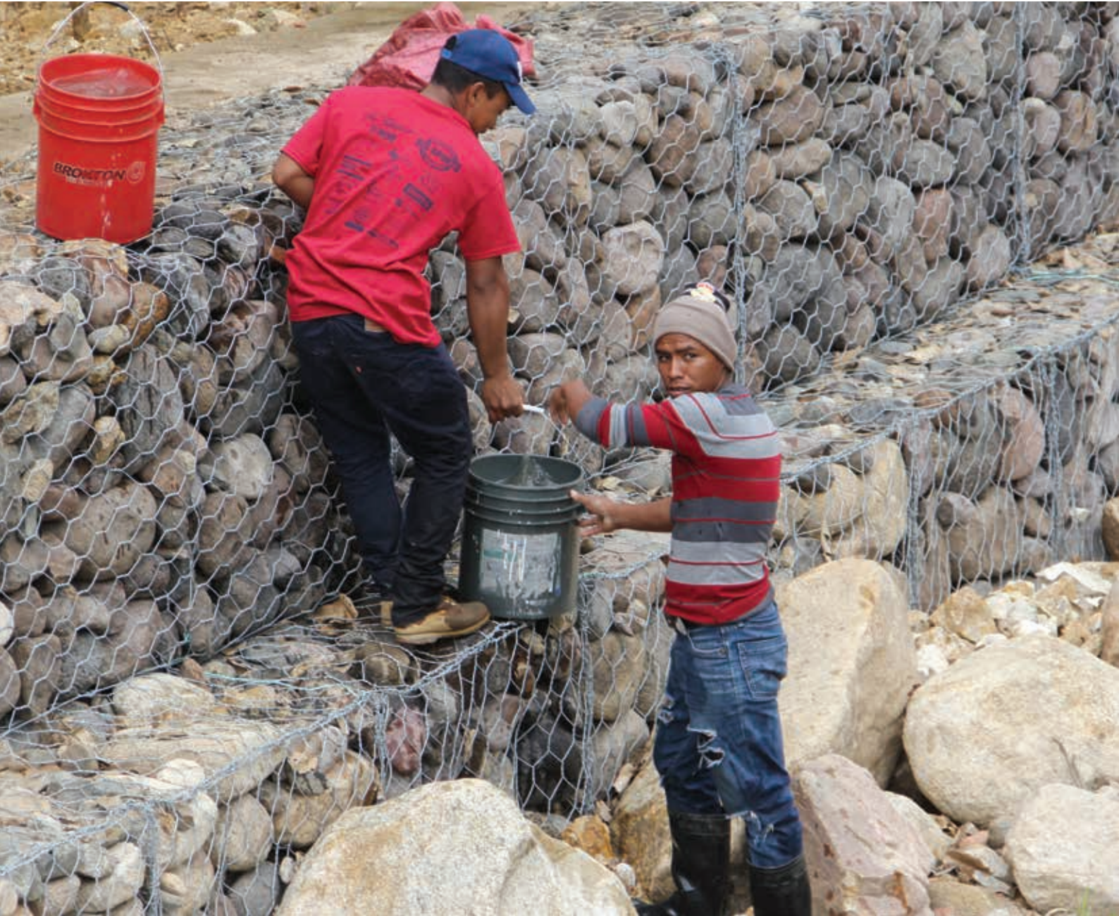
Maintenance works in tributaries of the Dipilto Basin, Nueva Segovia, Nicaragua. Photo: SDC.
